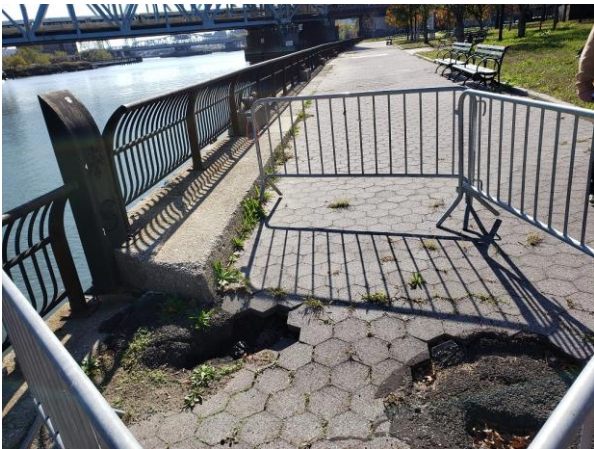
Greenway: Entrance to future park at 127 th /2 nd . Sinkholes- exhibiting effects of deteriorated bulkhead
