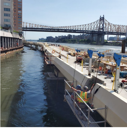
Parapet walls and preparation for closure pours to provide a continuous edge
