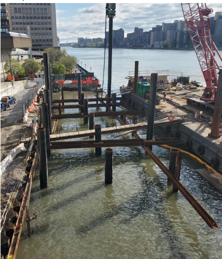
AHG caisson installation in the area where the existing platform has been removed
