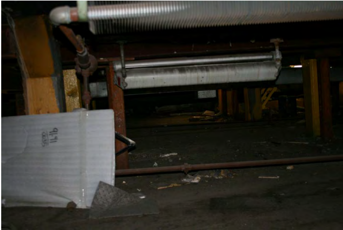
Photograph R: Four-foot deep service area beneath East Maintenance Area, facing east.
