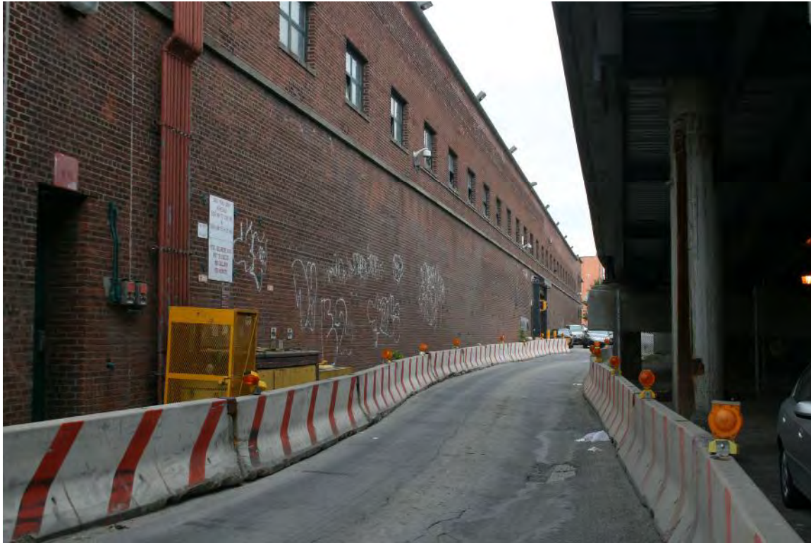
Photograph G: North elevation of 126 th Street Bus Depot facing west on 127 th Street.
