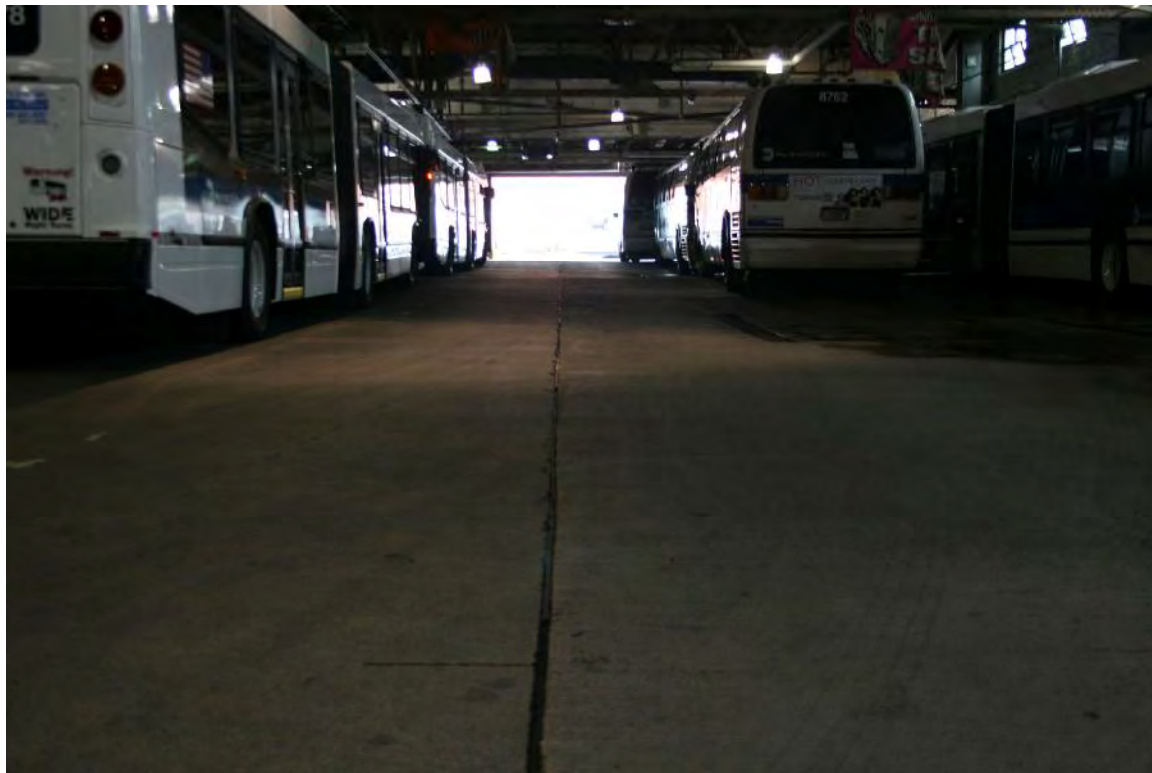
Photograph X: West end of Bus Wash where cement was piped below-grade ca. 2000 to raise the flooring which was sinking.
