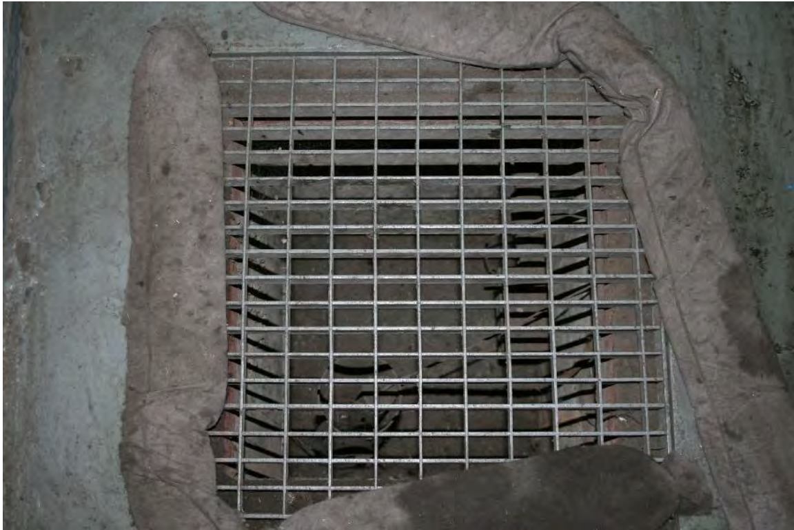
Photograph U: Grating in Pump Room floor over three-foot deep trench for piping.
