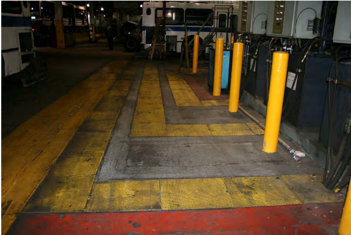
Photograph N: Power conduits from Lift Oil Tanks, ca.18 inches below grade, facing east.
