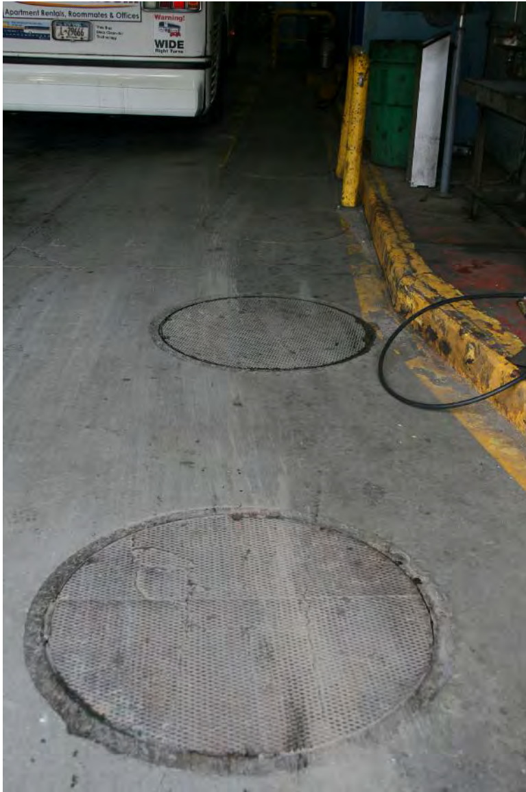
Photograph T: Location of original diesel tanks, now abandoned and filled, at southeast corner of building, facing north.
