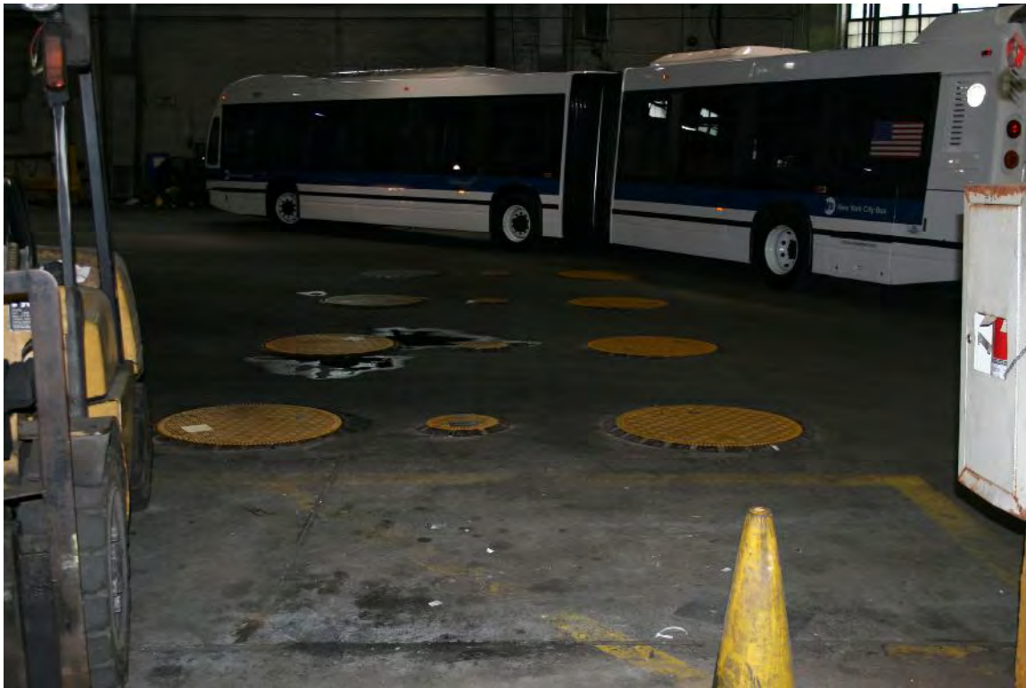
Photograph S: Eight 4,000-gallon diesel tanks, facing northwest. Each tank is six feet in diameter and excavated to ca.15 feet below grade.
