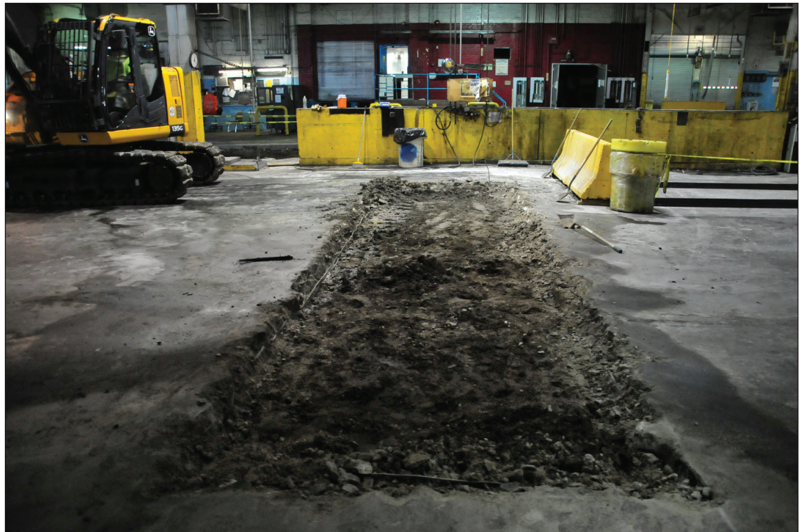
Facing south from bus wash area towards Trench 2 after concrete removal and before excavation 2
