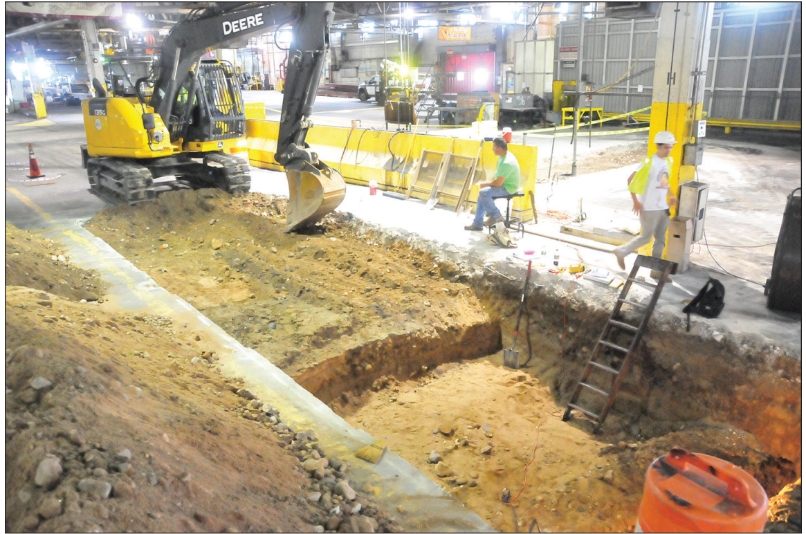
Facing northwest towards Trench 1 during excavation of west half; showing clean sands and gravel in the east half (at right) 5
