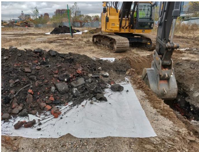
DEBRIS IDENTIFIED IN PETROLEUM IRM AREA
