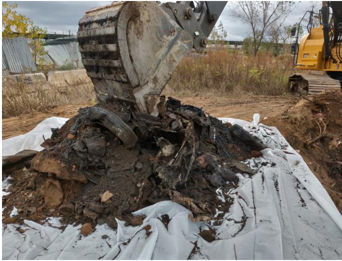
DEBRIS IDENTIFIED IN PETROLEUM IRM AREA
