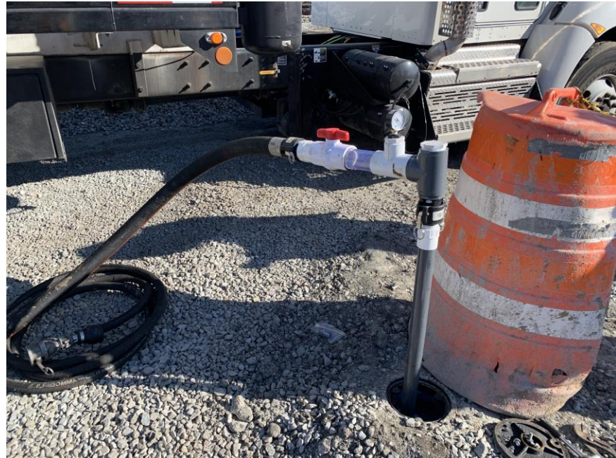
PRODUCT RECOVERY VACUUMING
