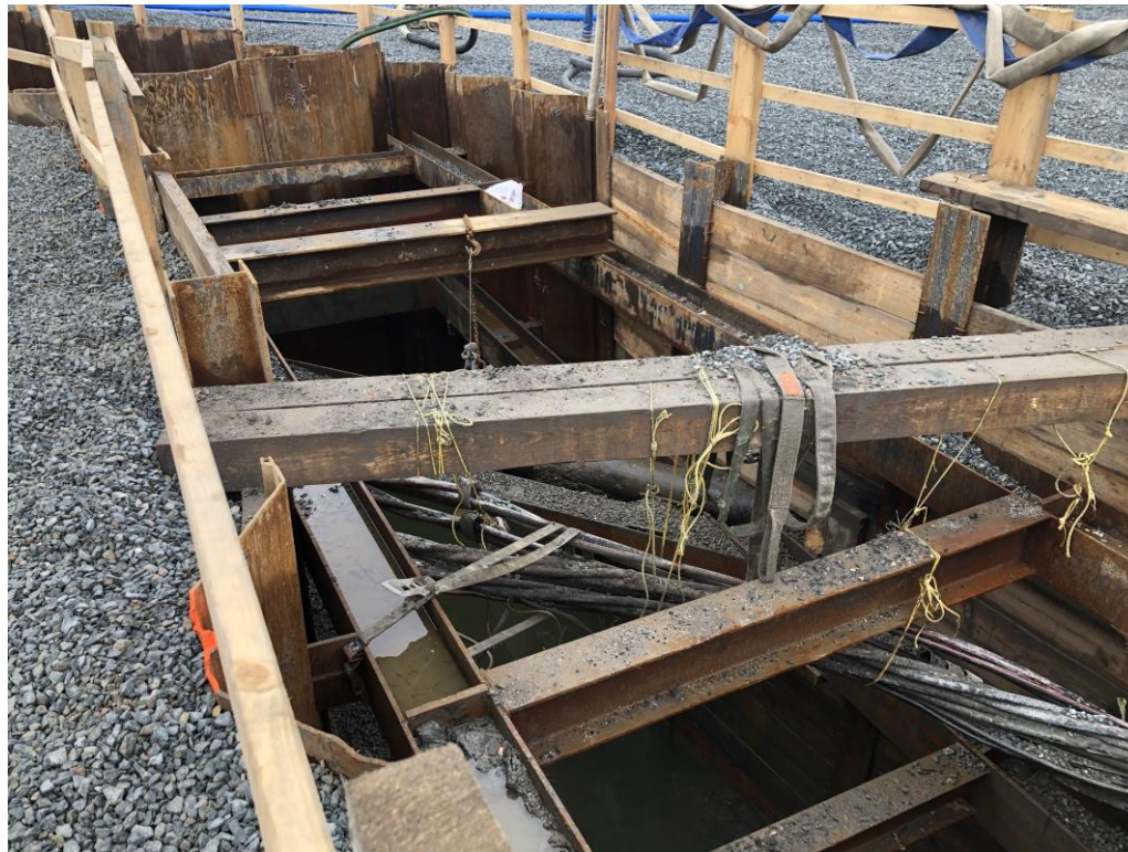
PROTECTED CONED INFRASTRUCTURE AT WATER MAIN CROSSING
