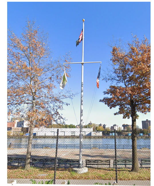
EXISTING FLAG POLE WITH YARDARM AND GRANITE BASE (x1) To be removed, refurbished, and reset in the original location
