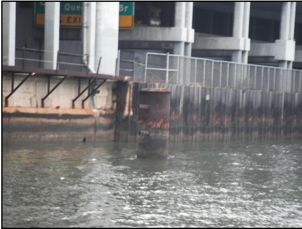
Photo 1: View of Concrete Facades and a Caisson from the Former Outboard Detour Roadway
