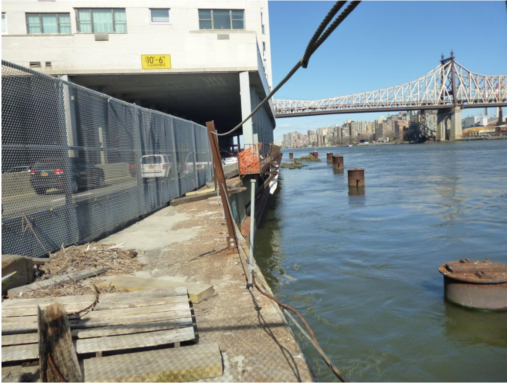
1 2 3 4 Photo 13 At end of existing esplanade looking north at fenced-off construction walkway along bulkhead adjacent to FDR Drive. Note building underpass and ODR drilled shafts/piles in river.
