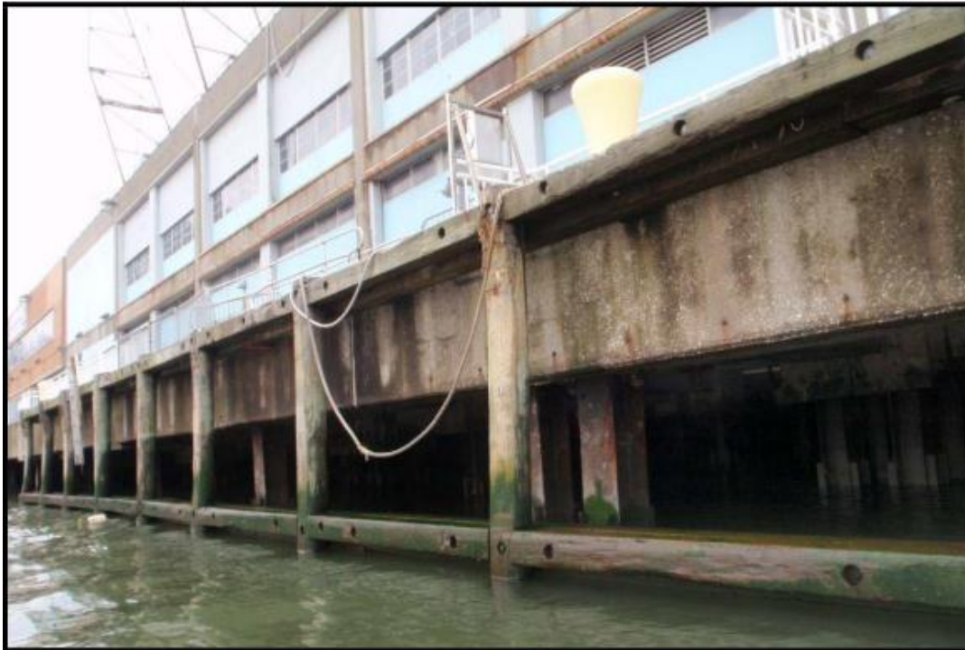
Photo 3: Pier 40. Note the numerous pilings and horizontal support members. Source: HPA Engineers P.C. 2009
