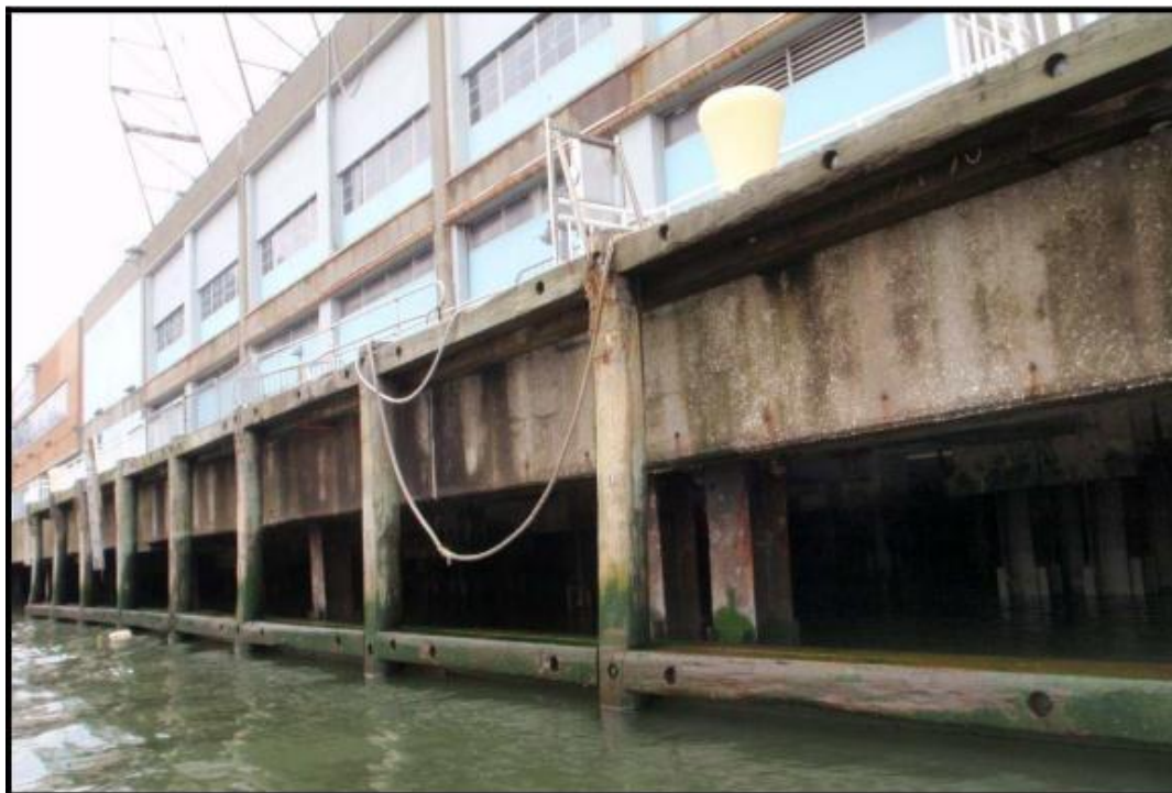
28 29 Photo 1. Pier 40. Note the numerous pilings and horizontal support members. Source: HPA Engineers 30 P.C. 2009
