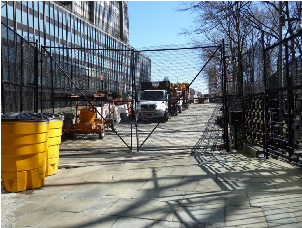
5 6 Photo 8 At northwest corner of UN property looking east at unused section of ramp adjacent to 7 north fence of UN property being used as construction equipment parking/staging area.
