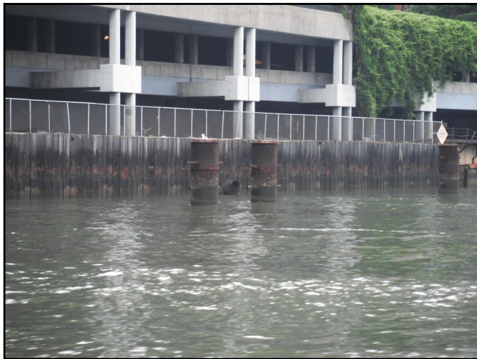
Photo 2: View of the Sheet Pile Bulkhead. Note outfall between the two caissons.
