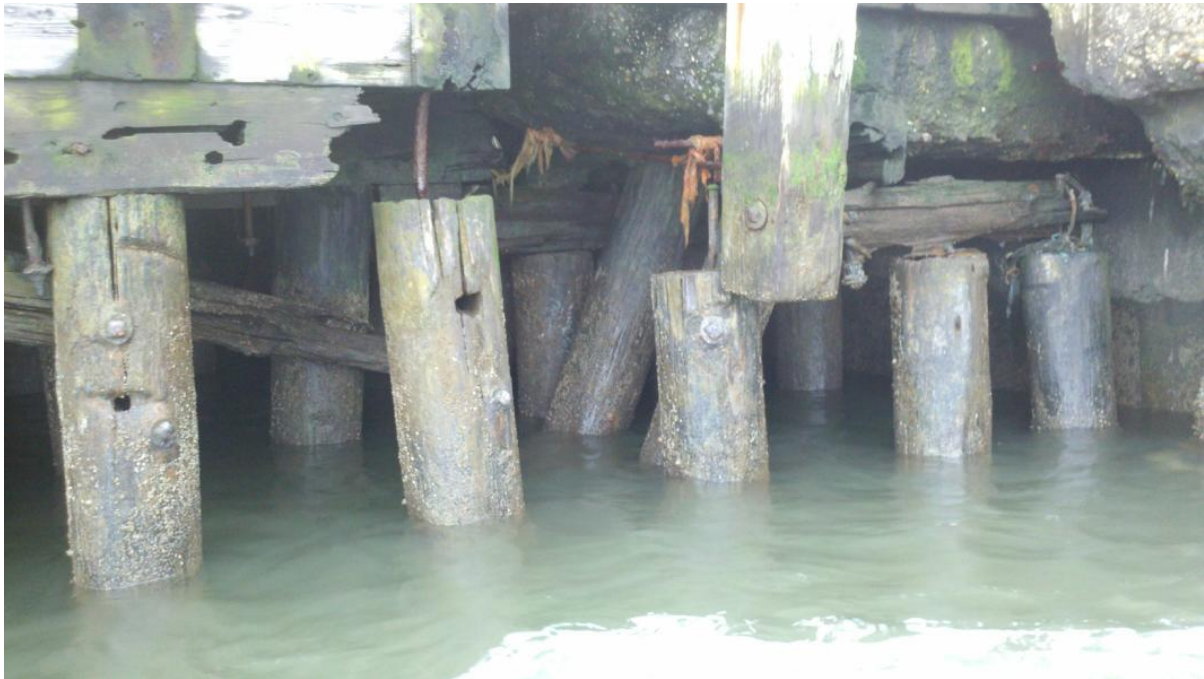
Photo 5 – Waterside Pier North Platform: Typical condition of pile cap – note completely eroded pile cap.
