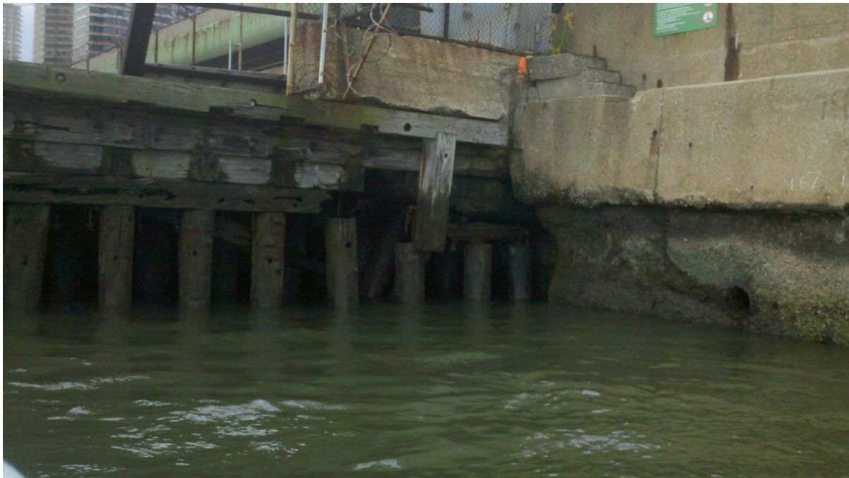
Photo 4 – Waterside Pier North Platform: Typical condition of pile cap – note completely eroded pile cap.
