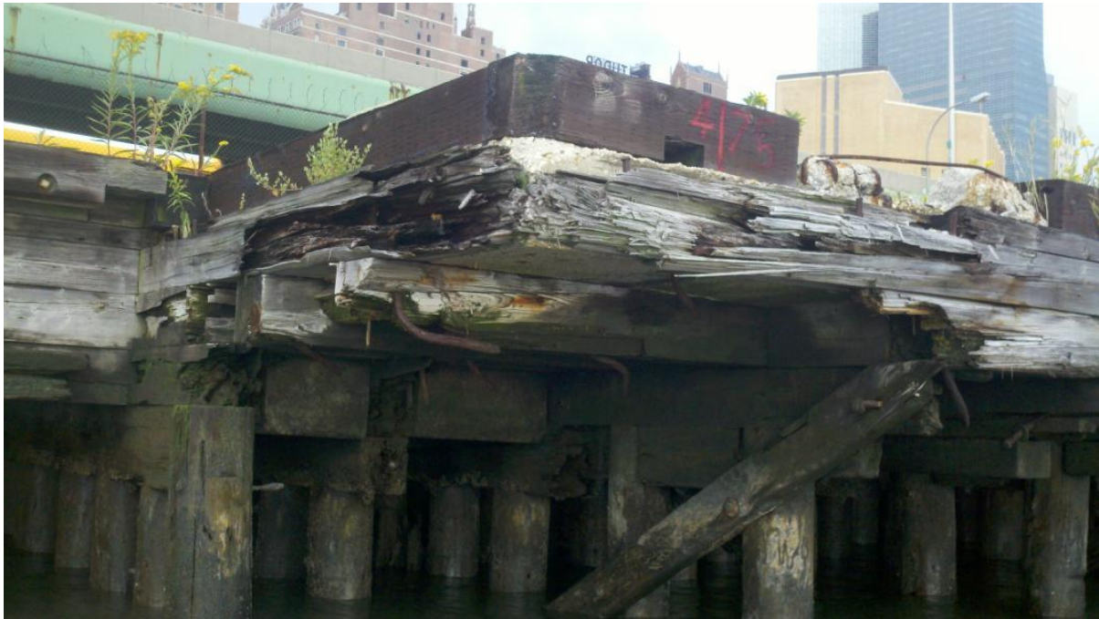
Photo 3 – Waterside Pier North Platform: Typical condition of timber fendering.
