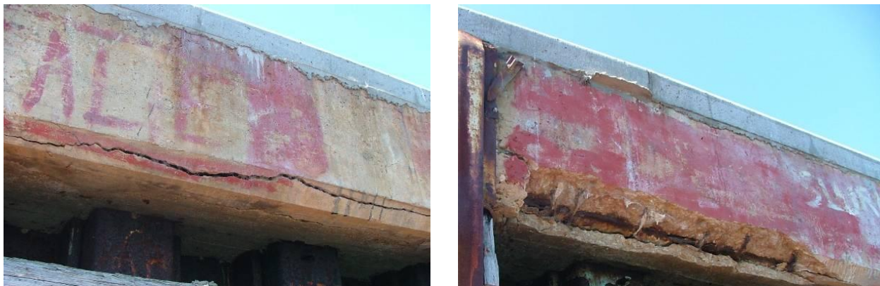
Figure 2-1: Examples of large cracking and spalling with exposed reinforcement as a result of chloride attack.
