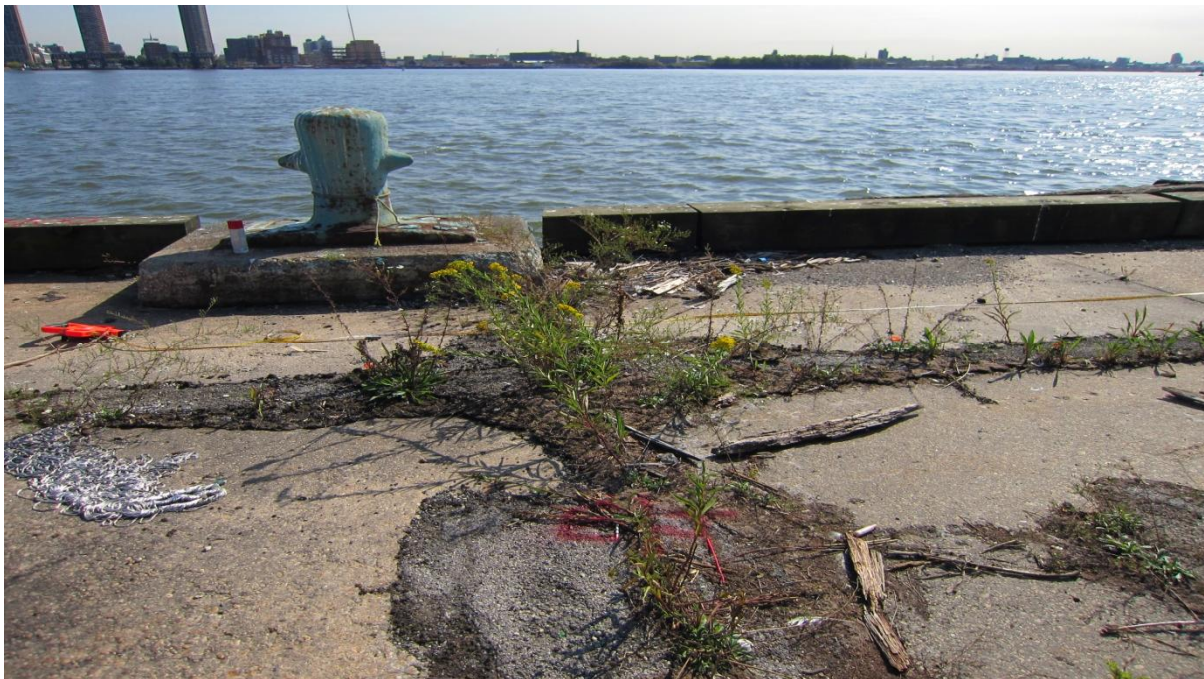
Photo 8 – Top of Platform with typical spall and vegetation
