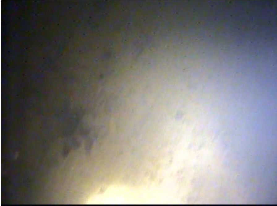
Photo 11– Waterside Pier Coal Pile measures 6 feet wide by 14 feet long, 4 feet deep located below the platform
