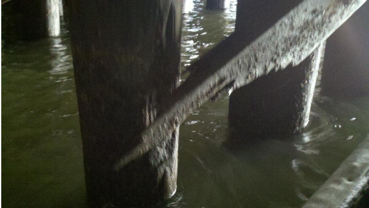
Photo 1 – Waterside Pier South Platform: Deteriorated timber bracing.
