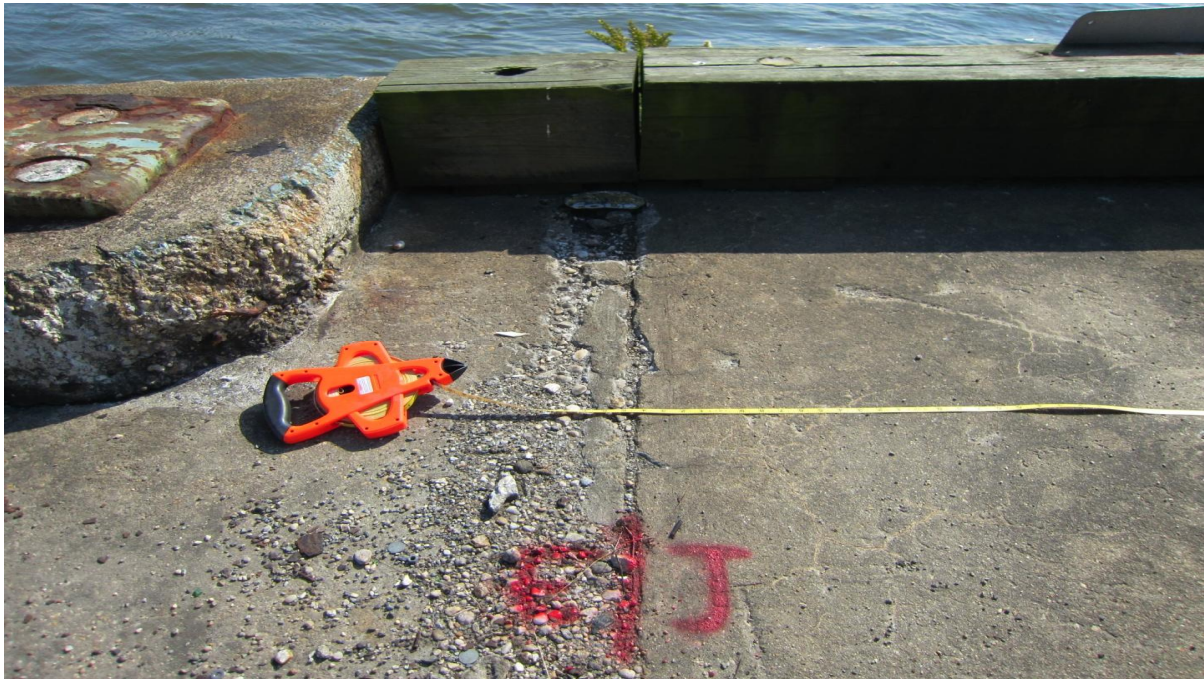
Photo 7 – Top of Platform with typical spall and delaminating
