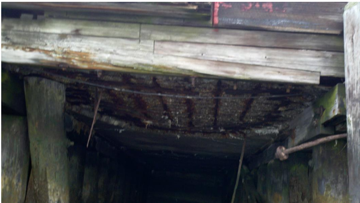
Photo 6 – Waterside Pier North Platform: Typical spall of reinforced concrete deck between bent rows.
