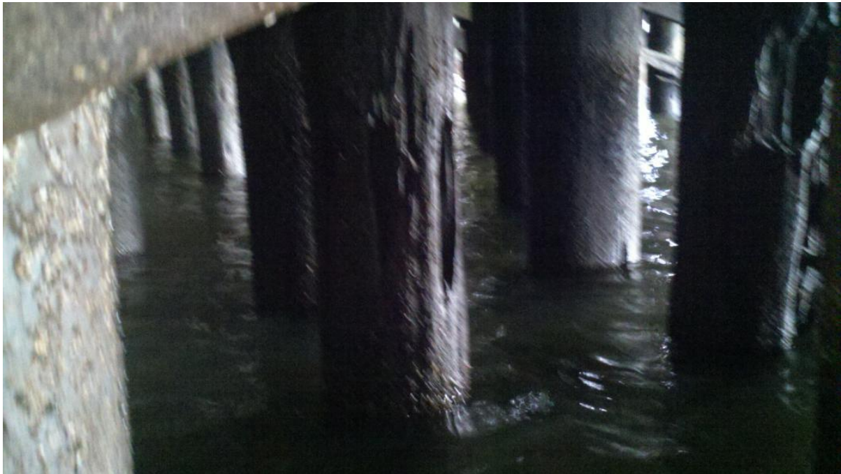
Photo 2 – Waterside Pier South Platform: Typical pile condition showing moderate to advanced deterioration in upper 6' to 8'.
